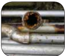
Corroded steel pipe
