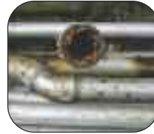
Corroded steel pipe
